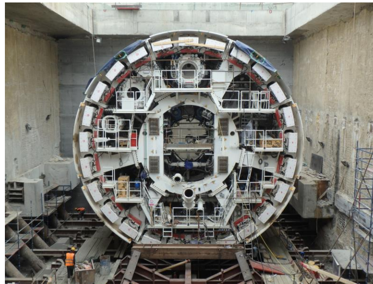
Ismailia Road tunnel – TBM Launch from two separate box shafts (anchored and strutted d-walls) for scheduling reasons
