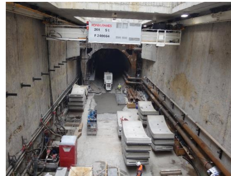
Nice (France) Tramway – TBM Launch from box shaft (anchored and strutted d-walls)
