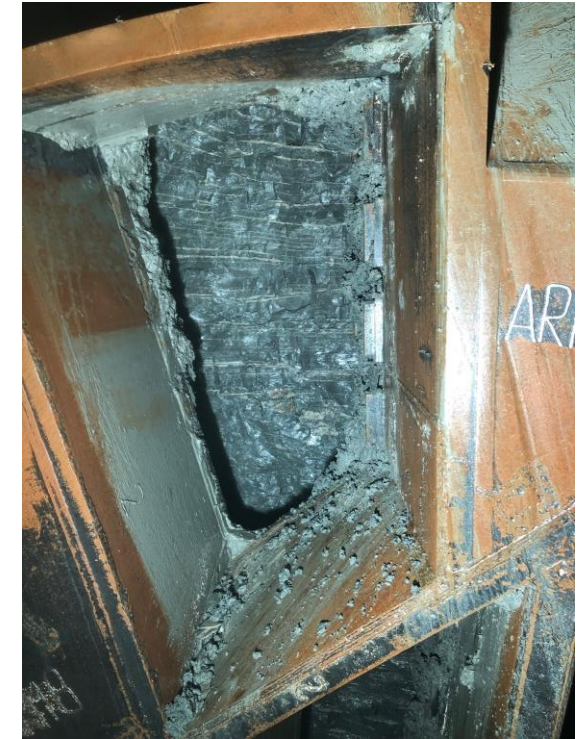
Face of the TBM in mudstone at Ahmed Hamdi tunnel. No clogging and dry face
